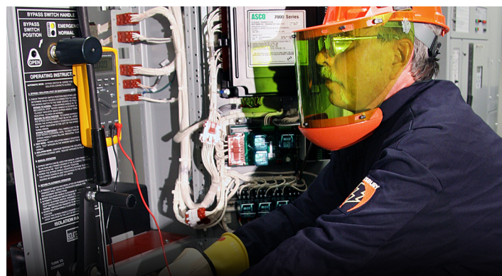
Service and maintain equipment without disrupting power to loads.
